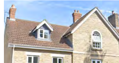
Gabled red clay pantile roof with exposed rubble façade and dormer window
