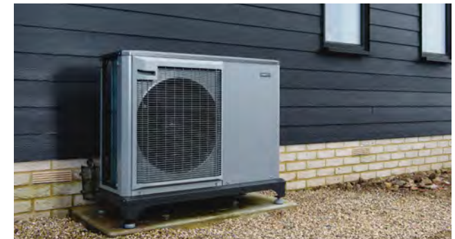
Figure 171: Example of an electric heat pump that is placed to the back of the house, whilst its grey colour fits nicely with the black weatherboarding of the property.
