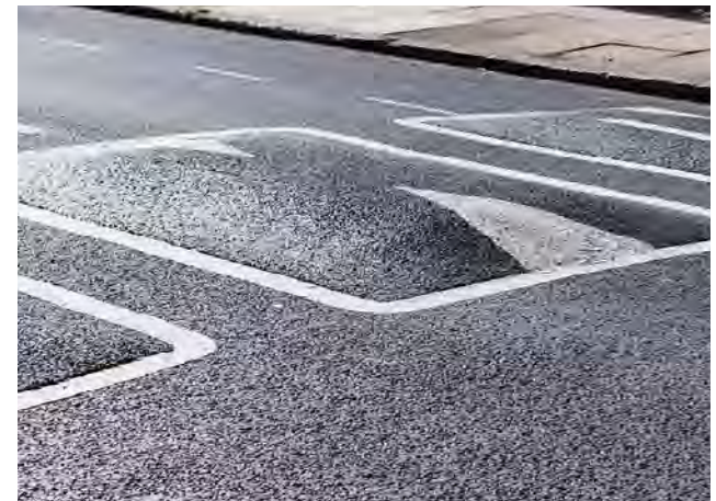
Figure 100: Example of a speed cushion.
