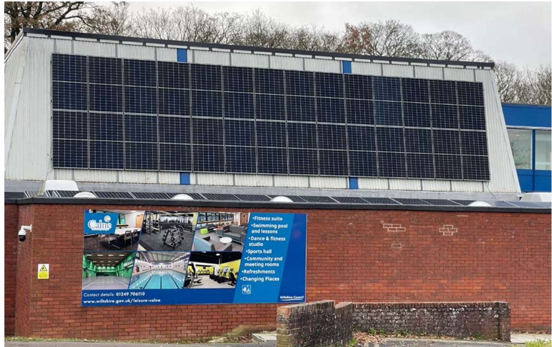
Solar panels at Calne Community Campus
