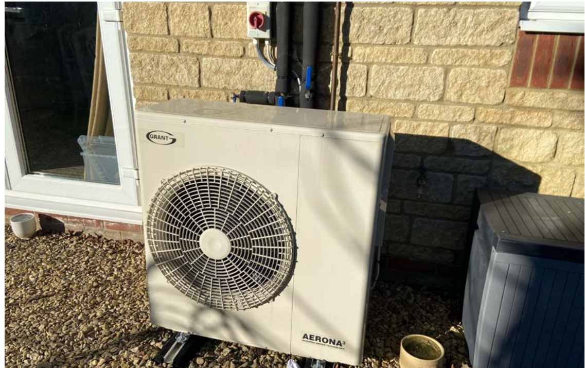
Domestic heat pump
