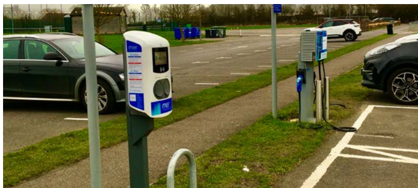
Charging points at Beversbrook Sports Centre
